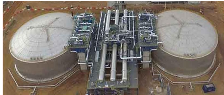
Molten salt tanks – hot and cold
